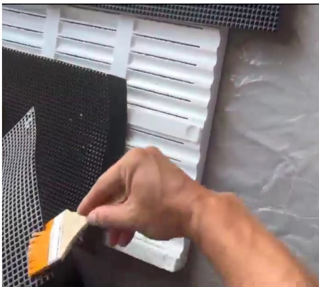
3- Use the brush to distribute the glue to the selected area, Put the Glue along the length of the mat roll with an area of 2-3 cm
